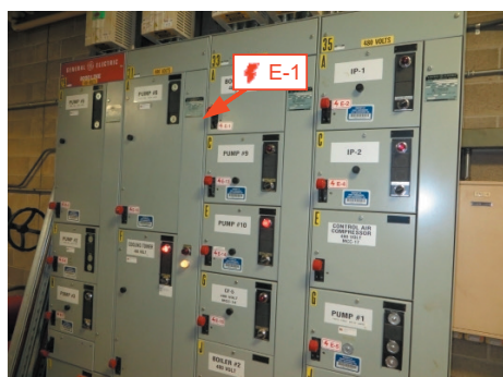
MCC 3 Column 3 Bucket A
